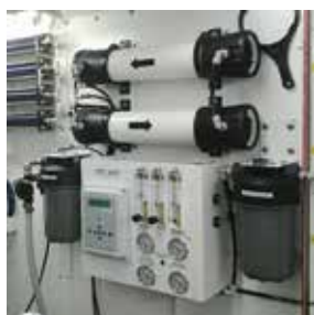
Dometic Spot Zero installed on-board.
